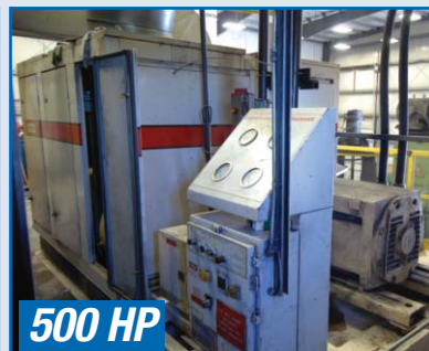
500 HP GARDNER DENVER AIR COMPRESSOR
